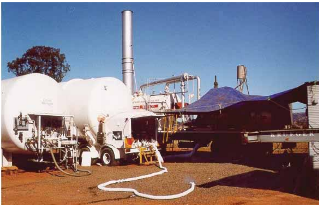
Figure 2.3 Mineshield inertisation unit on mine site
