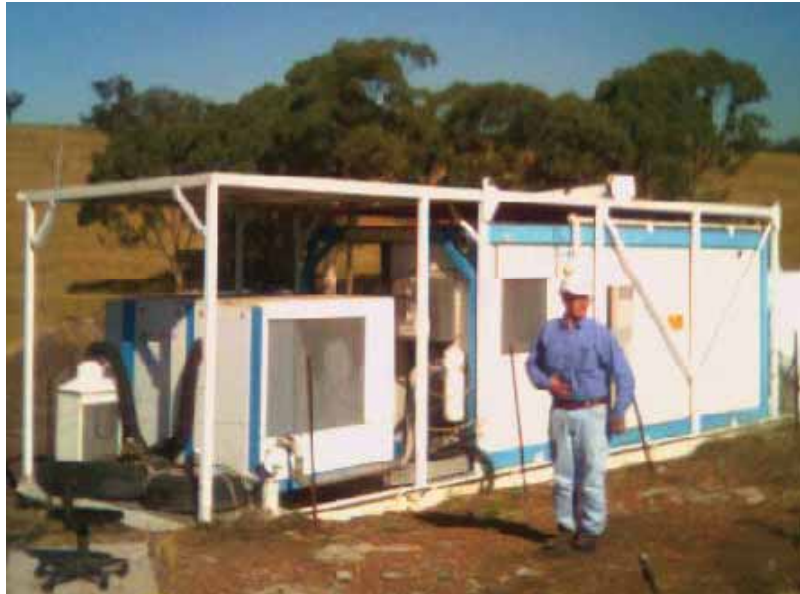
Figure 2.18 Floxal membrane inertisation unit at mine site
