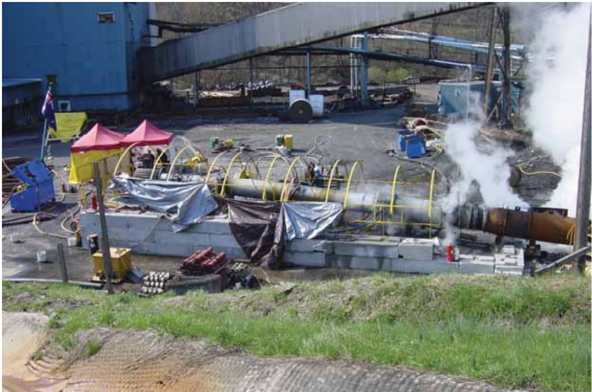
Figure 2.10 GAG-3A inertisation unit in use at the Loveridge mine, 2003
